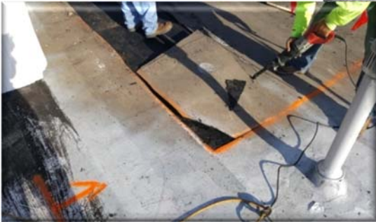
Wet insulation that had been identified during the moisture scan was removed from the roof system.
