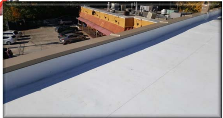
New Kynar finished coping metal was installed along the parapet wall. The standing joints were folded together and sealed to make leaking almost impossible.
