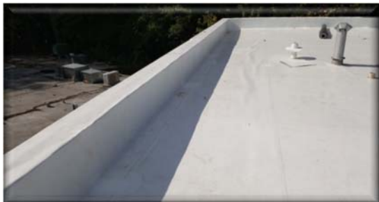
60 mil white TPO membrane was then installed and also secured with plates and screws. The seams were heat welded together to form a "continuous" envelope for the roof.
