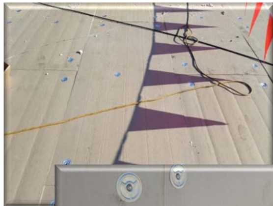
New mechanically fastened insulation with an R-value of 20+ to meet code and tenant demands was installed.
