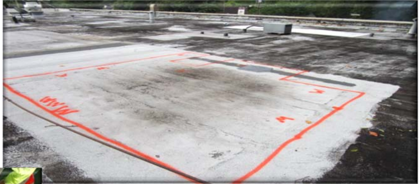
Roof inspection revealed wet insulation.
