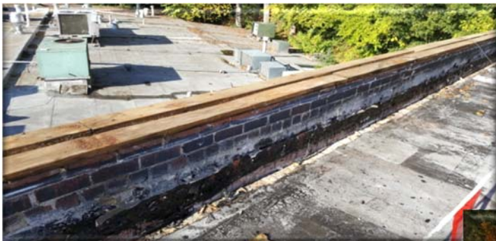
A new wood nailer was added to the top of the parapet wall at the perimeter of the building to accommodate new preformed coping metal.
