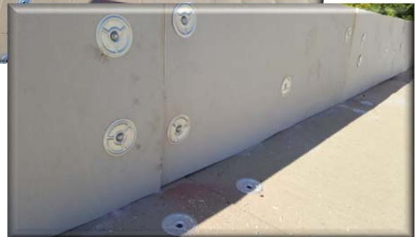
New insulation was also added to the side and top of the wall to provide a smooth roofing surface.
